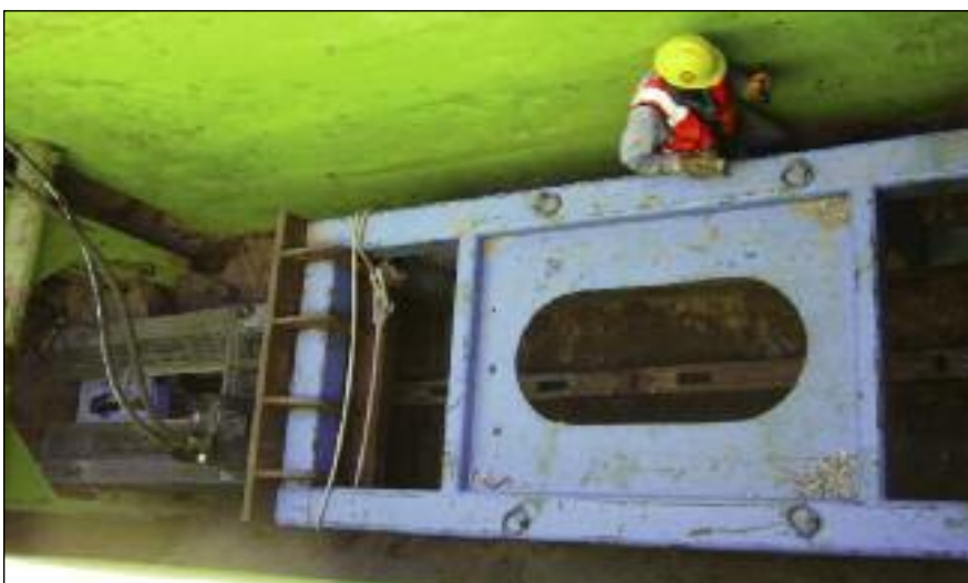
GrundoburstR 2500G and extraction cage in receiving pit
