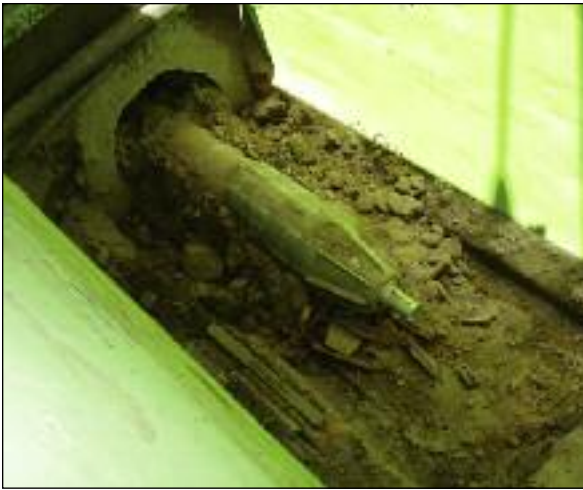
24 inch OD expander followed by new 18 inch VCP jacking pipe on arrival into the receiver
